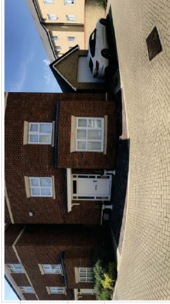
UNLAWFUL ALTERATIONS TO APPROVED SCHEME (AS BUILT)
